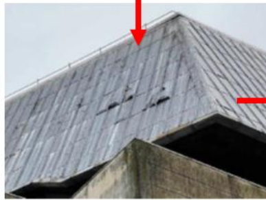
Vertical lead clad mansard surrounding the roof area, visible from street level
